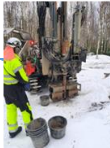
Drill sampling of the Korsnäs historical Tailings Storage Facility (TSF) commenced February.
